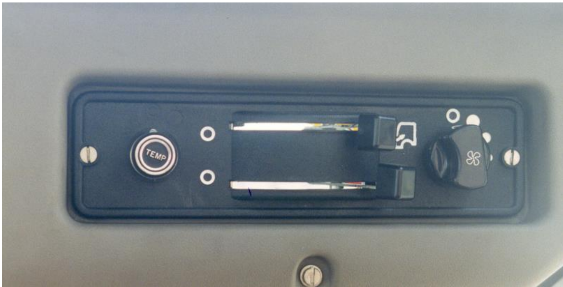
Thermostat location on panel.
