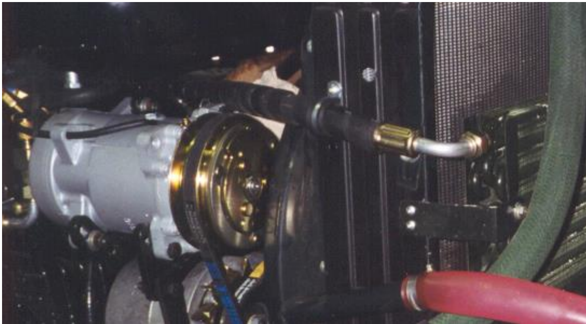
Discharge line routing showing clamp on radiator frame and connection at condenser.
